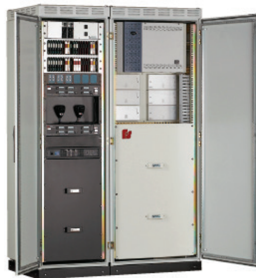
Rack Mounted ECHO System
